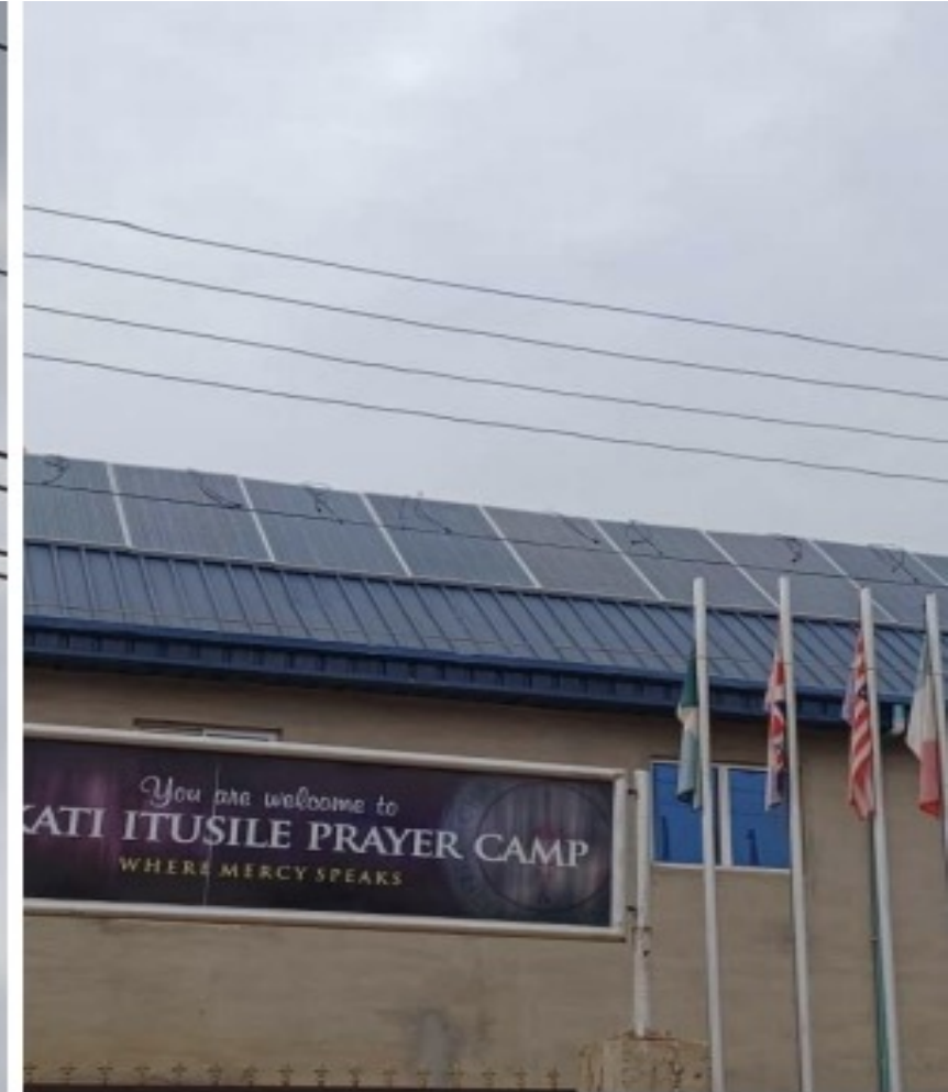
10KVA INSTALLATION AT WAKATI ITUSILE PRAYER CAMP
